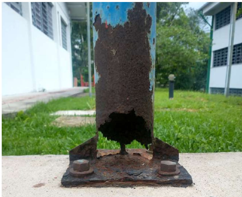
Figure 1 – Effects of corrosion. Source: Author
